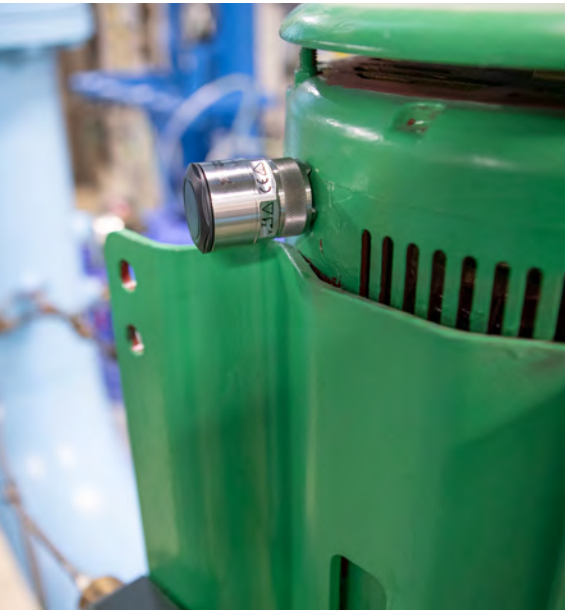
Figure 4: MEMS-based sensor connected to a vertically installed motor wirelessly sends data to experts for analysis
